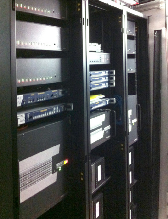
Three XTP CrossPoint matrix switchers and a variety of FOX Series fiber optic extenders from Extron provide AV signal switching and distribution throughout the shopping complex.
