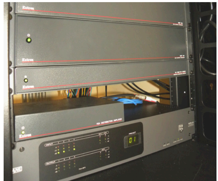
Equipment Rack with Extron P/2 DA4xi and DA4 RGBHV Distribution Amplifiers and WindoWall Processors
