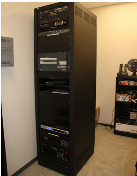
The XTP CrossPoint and shared resources are rack mounted within an equipment room adjacent to the pre-function area.
