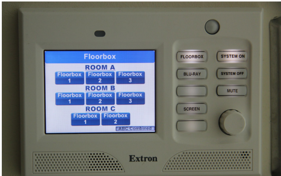
When all partitions are removed to form one large presentation space, the Extron TLP 350MV in Training Room B provides AV system control in a small affordable package.
