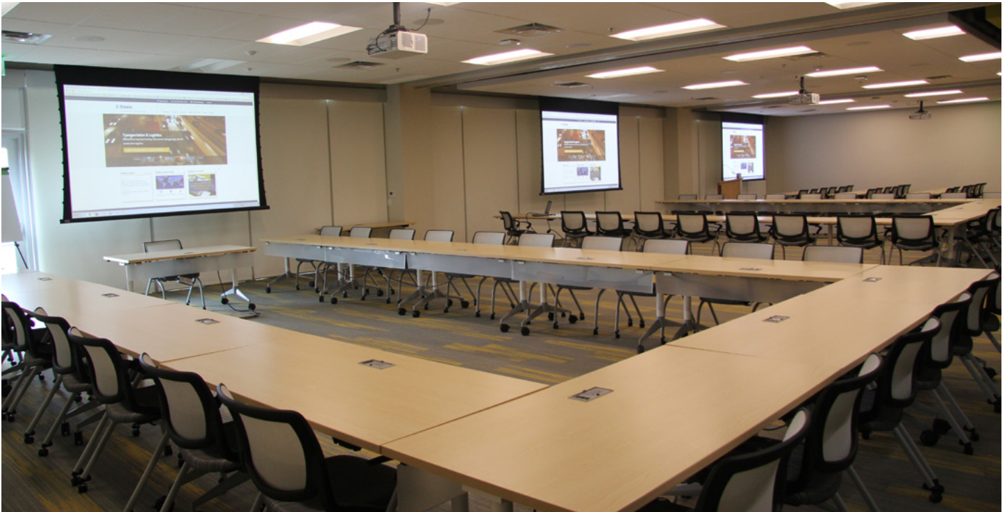
An Extron XTP CrossPoint 1600 matrix switcher in the divisible training room provides AV switching flexibility to meet any room configuration.
