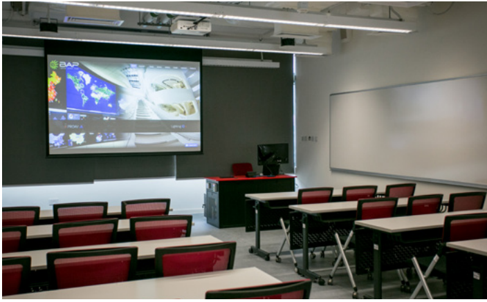
There are 14 standard classrooms equipped with identical AV systems for a consistent look and feel. Instructors can enter any classroom and start the AV system in seconds to get the lesson plan underway without delay.
