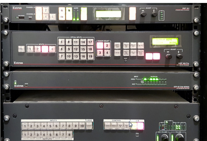
To stream and capture content from presentations and the various video sources, an Extron SMP 351 is mounted in each room's equipment rack.
