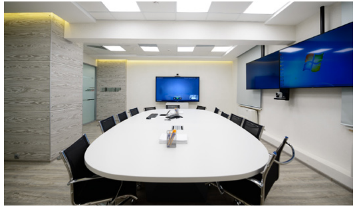
For remote displays in larger spaces, signals are extended using Extron DTP HDMI 4K 330 Series transmitters and receivers. Photos courtesy of SIBUR.
