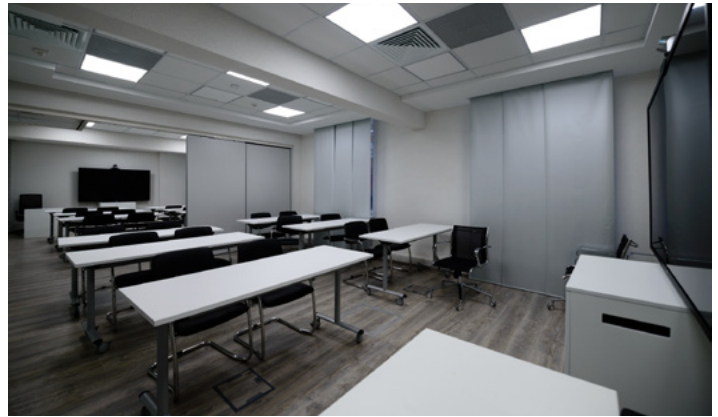
To facilitate AV signal switching and distribution of 4K video resolutions over HDMI, a DTP CrossPoint matrix switcher is installed in each room's credenza. Photo courtesy of SIBUR.
