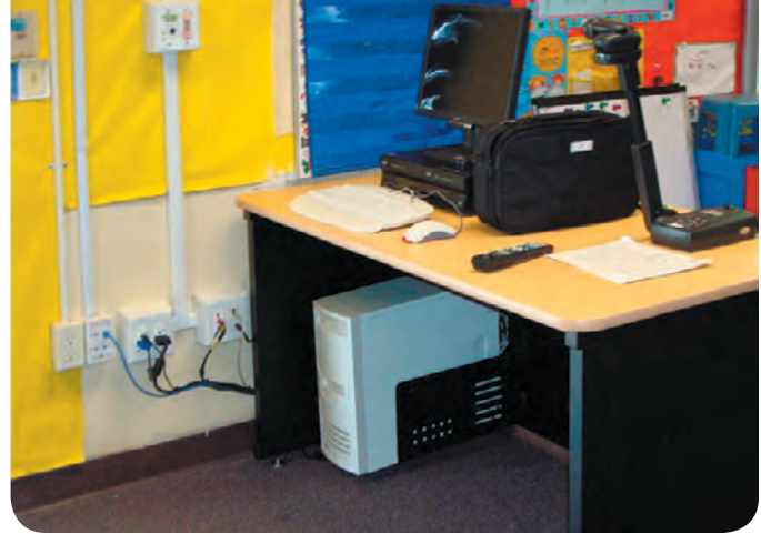
A/V connections and the system control panel are easily accessible from the teacher's workstation.
