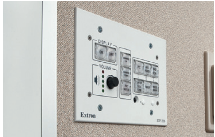
Each classroom features two easy-to-use MediaLink controllers, allowing the teacher to control the classroom AV from the front or back of the room.
