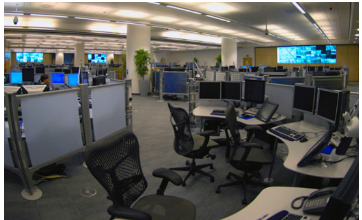
Three videowalls were installed at this Special Operations Centre in Lambeth, one of three such facilities for the Metropolitan Police Service.
