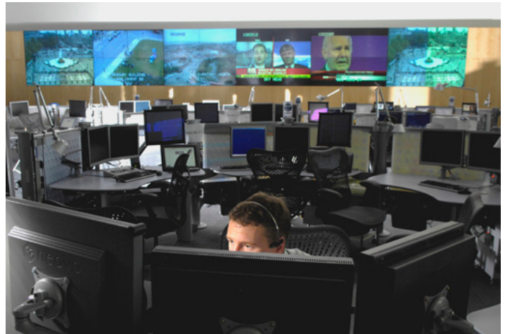
The Metropolitan Police Service employed videowalls to make surveillance camera feeds and other information readily viewable by many staff members.
