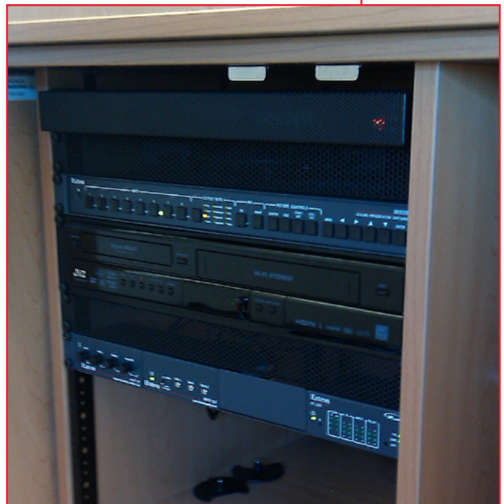
The rack mounted Extron IN1508 and IPL 250 provide scaling, switching, and Ethernet control
