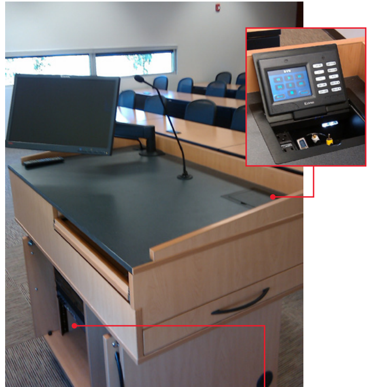
The TLP 350CV touchpanel mounted on the podium provides room control and AV connectivity
