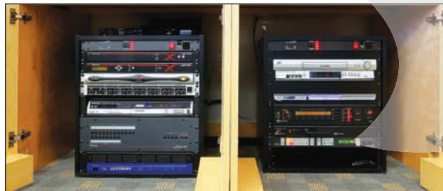
Rack equipment for the conference room, with the Extron MGP 462 dual window processor and CrossPoint 300 128 HVA matrix switcher
