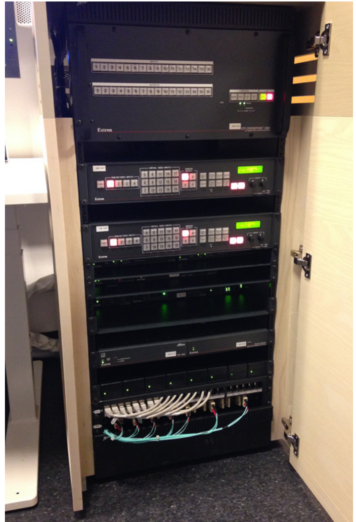
The AV equipment room is used for monitoring and supporting the amphitheater AV system as well as content distribution to the dissection rooms.
