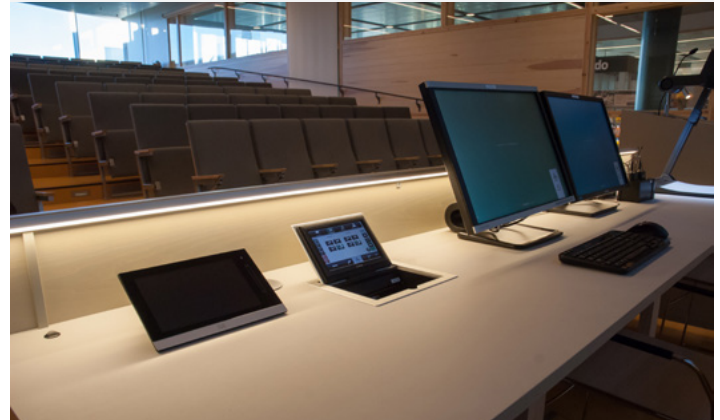
A TLP 710CV touchpanel in the auditorium allows instructors to quickly and easily operate the AV system, including available videoconferencing functions, from the instructional table.
